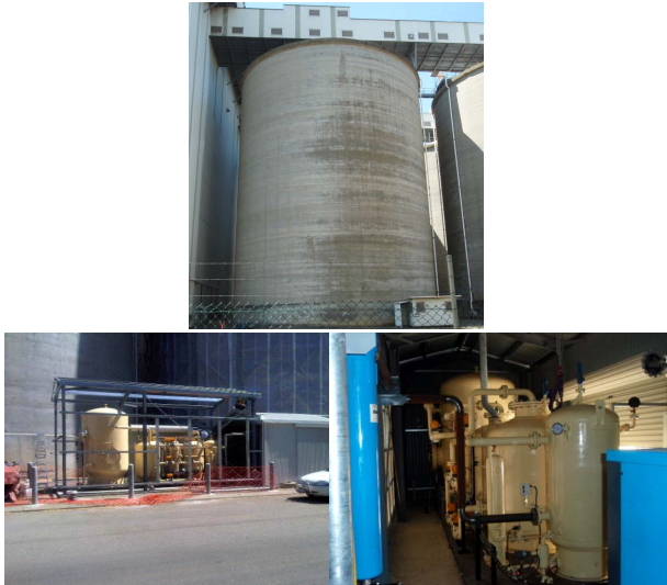
Fig.3 A 350 m 3 /hour PSA nitrogen generator has been installed at the CBH Albany grain export terminal (35°1'50.90"S 117°53'10.54"E). The generator is plumbed to a bank of 10 × 10,000 tonne concrete cells.
