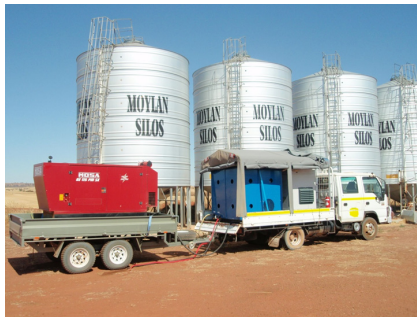
Fig.2 Nitrogen application underway to 75 tonne silos. This Membrane Nitrogen generation unit (60 m 3 /hour, 99% pure nitrogen) is completely mobile being powered by a diesel generator.
