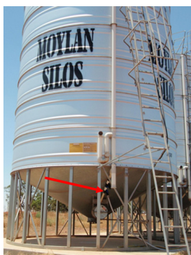
Fig.4 Tap system installed in existing thermosiphon pipework. Thermosiphon pipework consists of 90 mm stormwater PVC pipe leading from headspace of silo to ground level phosphine application chamber. Phosphine chamber has entry duct into base of silo, to complete the recirculation loop.
