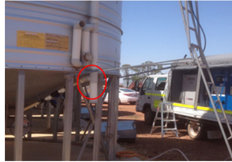
Fig.5 At the join of the cone and sidewall of the silo, the thermosiphon pipe reduces in diameter to 40 mm Drain and Waste (DNW) pipe. This reduced diameter pipe connects with the ground level phosphine application chamber. It is this pipe where the Nitrogen application tap system was installed into.
